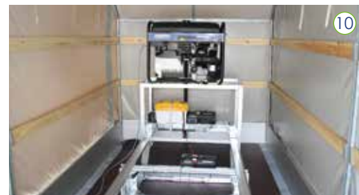
The equipment is connected to - and powered from - the onboard generator located inside the trailer.
